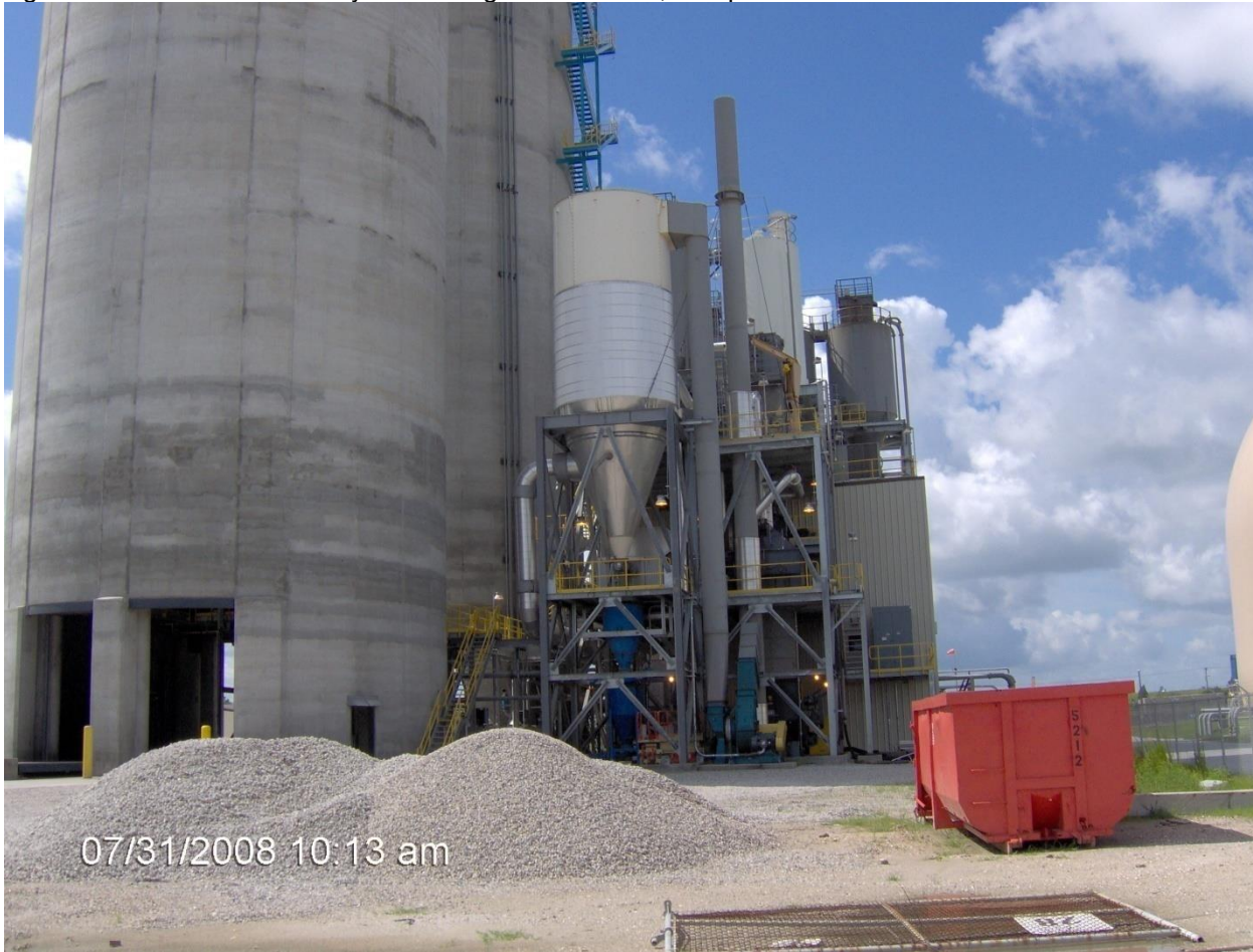
Figure 2: Ammonia removal system at Big Bend Station, Tampa Florida
